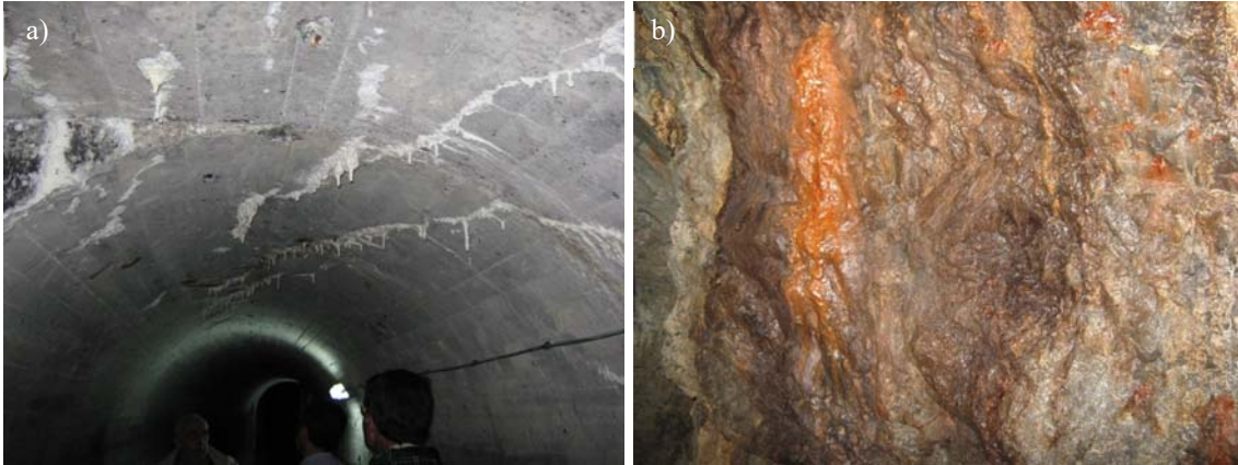
Figure 12. a) Oblique cracks in an upper gallery near the left abutment (level 1350 m) and b) state of the rock in the right abutment seen from the second gallery (level 1330 m).
