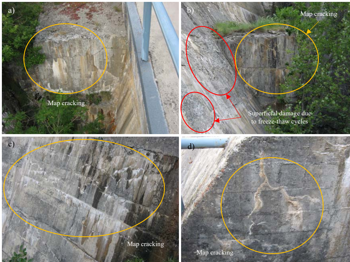
Figure 11. Map cracking localized in specific areas of the dam: a) block beside the right abutment, b) block beside the left abutment, c) downstream face and d) entrance to the upper gallery.
