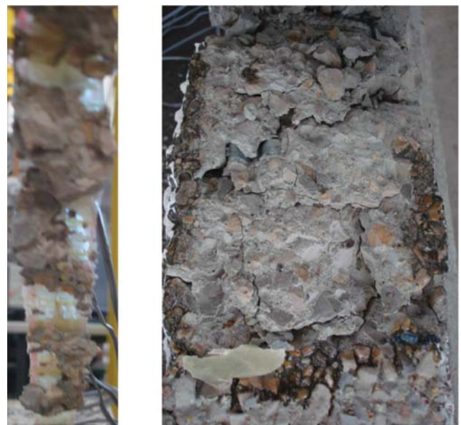
Fig. 12—Failure surfaces after 10,000 hours. Cycles -10 and 30°C (14 and 86°F). Strips 20 and 80 mm (0.787 and 3.150 in.).
