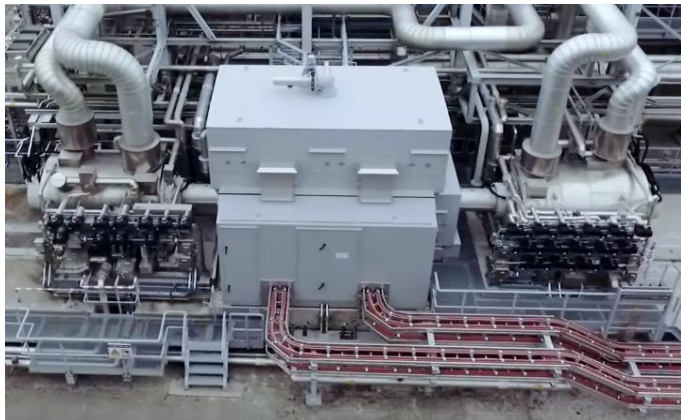
Figure 2. 23-MW (30,000hp) Direct Driven Compression String with Synchronous Motor in Double-End-Drive Configuration, Schaapbulten, Netherlands
