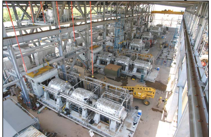
Figure 21. Photograph of Compressor Deck showing the Six Compressor Strings. From front to back- 2 x Methane compressors, 2 x Ethylene compressors and 2 x Propane Compressors.
