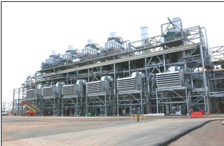
Figure 5. Gas Turbine Compressor Trains with Four Heat Recovery Units (OTSGs) on the left.
