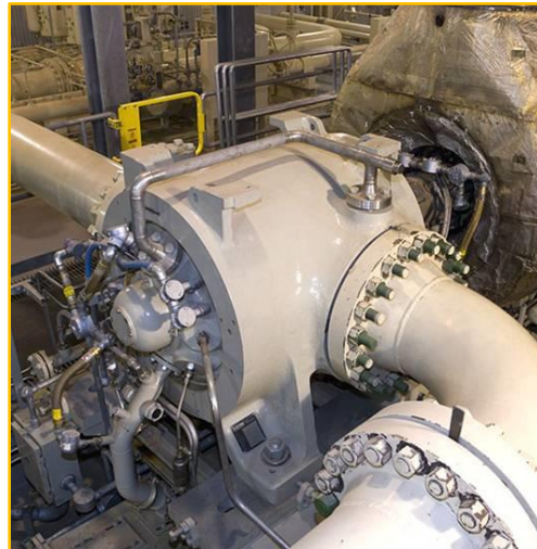
Figure 1. Compressor model at a site installation and driven by a gas turbine engine
