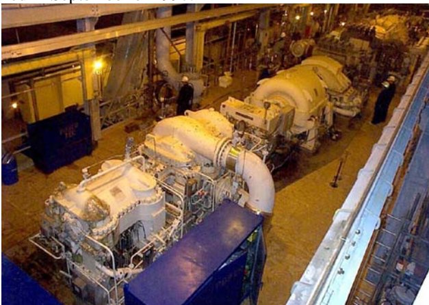
Figure 7. Photograph of DuPont's charge gas train.
