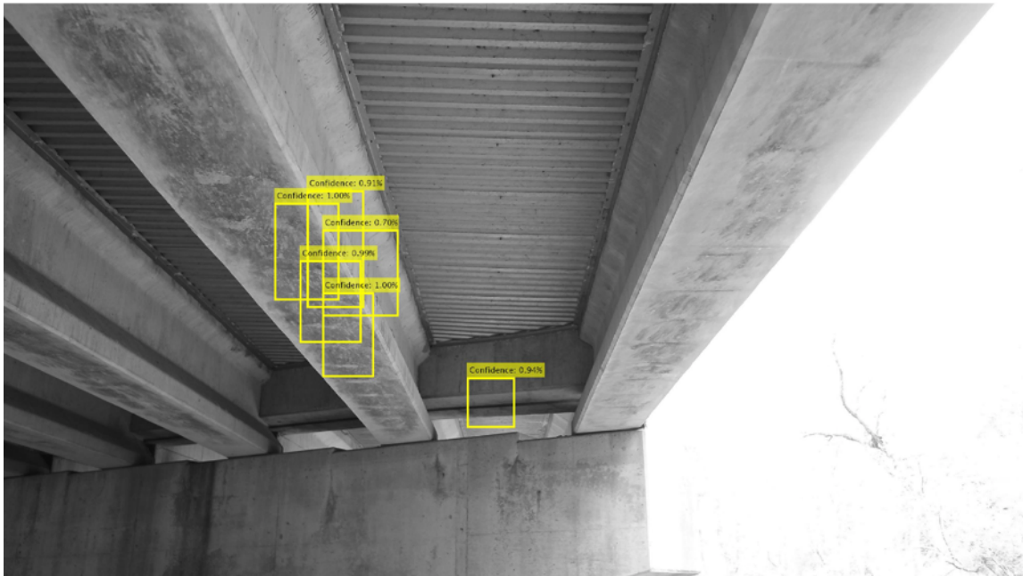
Figure A - 2. Beam flange false positive: Example 2
