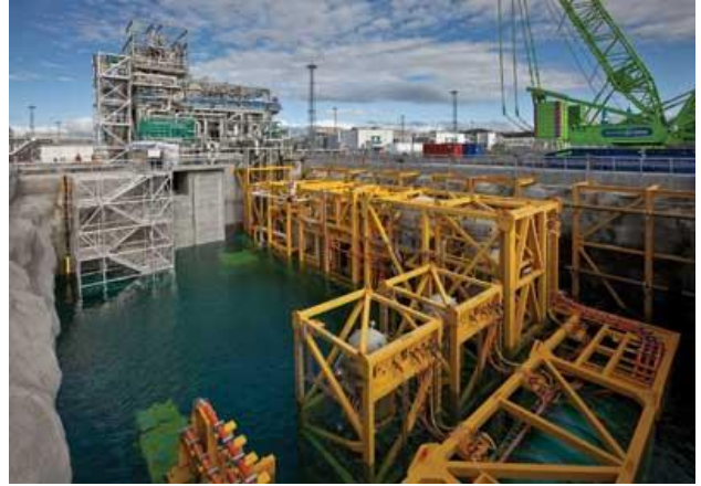
Figure 3: Extended Factory Acceptance Test in the pit at customer facility in Nyhamna, Norway
