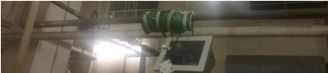
Figure 21. Installed flowmeter on the 2" main header line.
