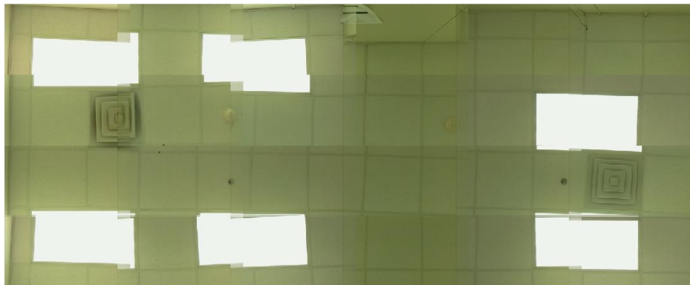
Figure 55. Demonstration of image stitching using known locations. In the proposed system, the known locations come from navigation and exploration information.
