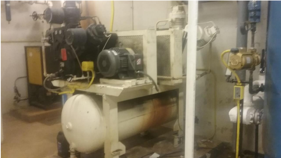
Figure 20. Compressed air system used in field test.
