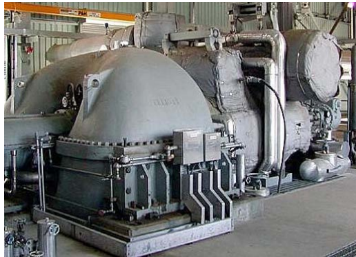
Figure 10: Steam Turbine Exhaust
