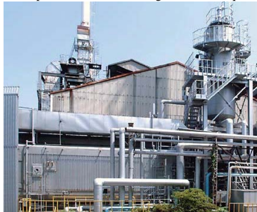
Figure 34: Boiler for Steam Turbine Test, Courtesy: Hitachi
