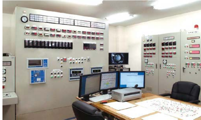
Figure 33: Steam Turbine Test Control Room - Courtesy: Hitachi
