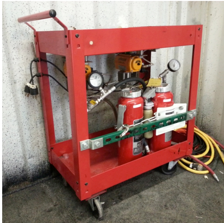
Figure 20 - Complete fire extinguisher cart.
