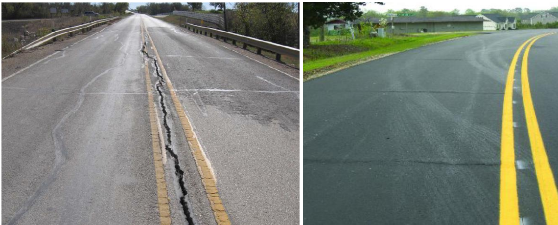
Figure 4. Instance of Longitudinal Cracking and Transverse Cracking. Reprinted from
