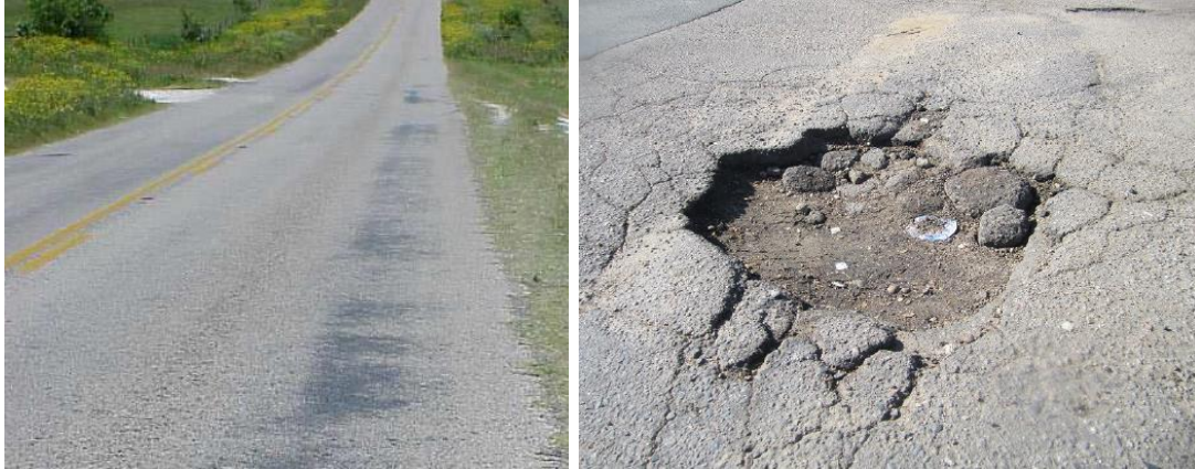
Figure 5. Instances of Ravelling and Pothole. Reprinted from [7].
