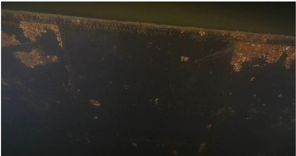
Figure 9.14- A panel with relatively no corrosion nodules in between areas with corrosion product patches. Note the straight lines following the seams. Photo by Kees Beemster Leverentz.
