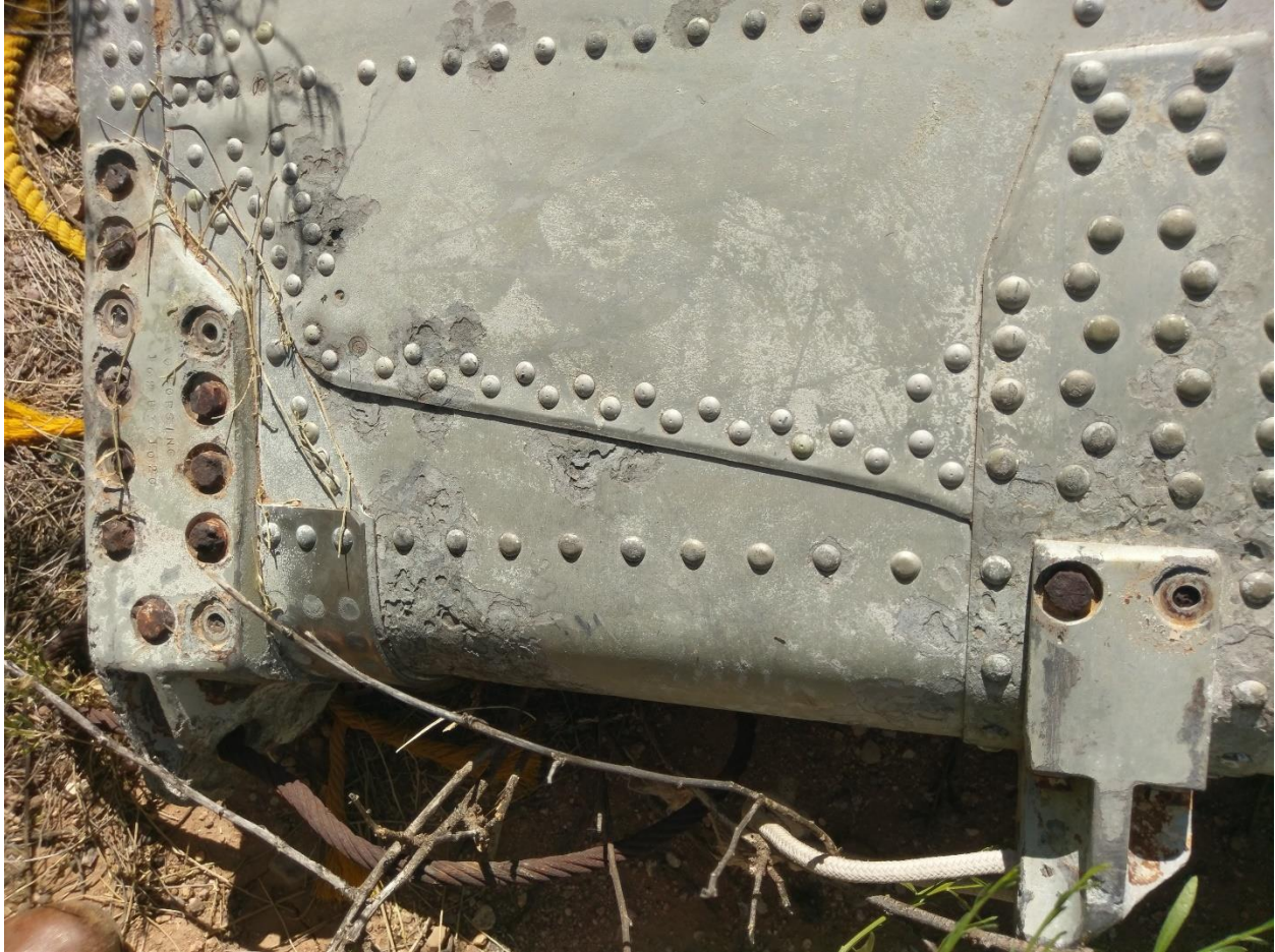
Figure 9.35- Corrosion pitting damage to the rear afterbody as seen in 2018. Note the bare metal has a slight hint of green primer and the pits do not appear to go all the way through the reinforced aluminum in this area. Photo by the author.
