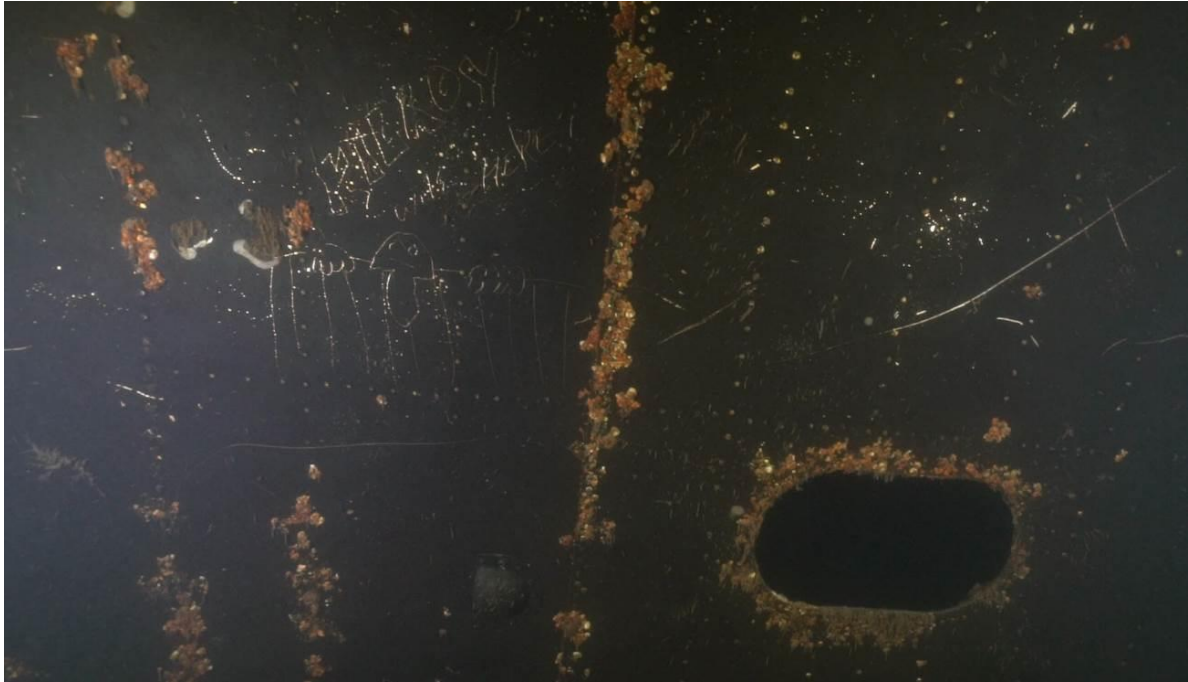
Figure 9.13- Corrosion patterns following rivet seams and the outline of a window, but does not affect every rivet seam. Note the graffiti on the top left. Photo by Kees Beemster Leverentz.
