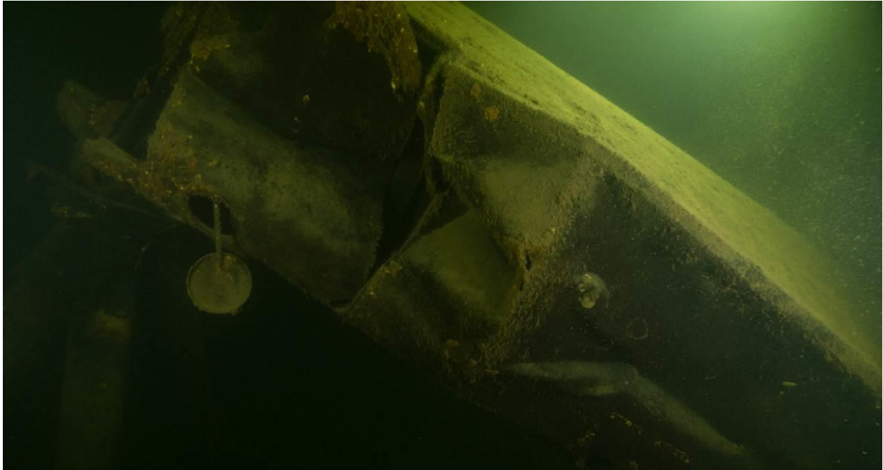
Figure 9.8- Part of the damaged port side pontoon float. Photo by Kees Beemster Leverentz.
