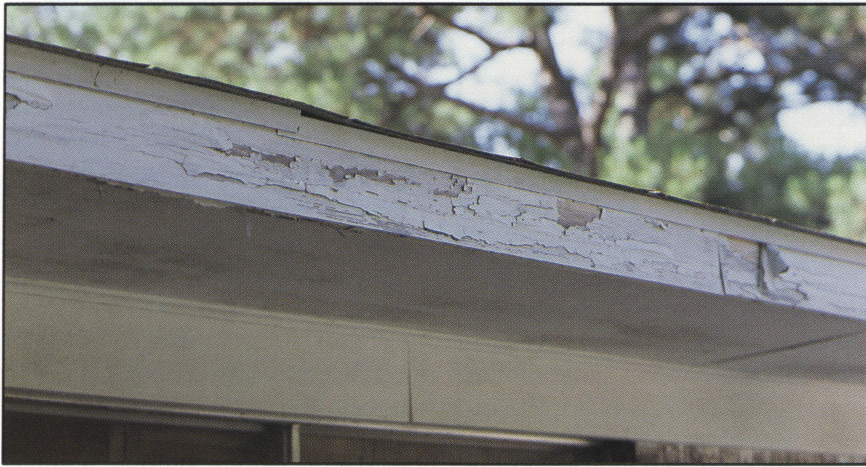
Southern pine trim not treated with a water repellent and painted with oil-based paint quickly fails.
