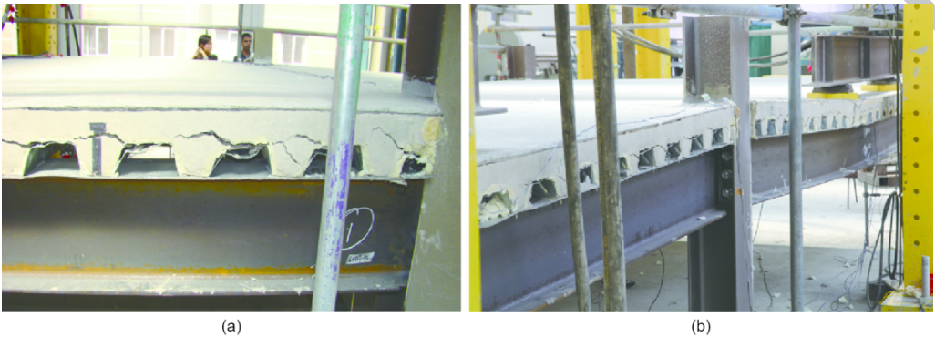
Fig. 19. (a) Crack at the edge of the slab without U-bars at failure, and (b) deflection of the edge beam with U-bars.
