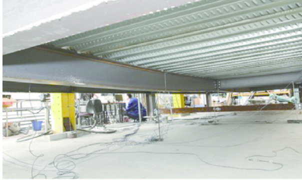
Fig. 12. Deflection of internal secondary beams at maximum load.
