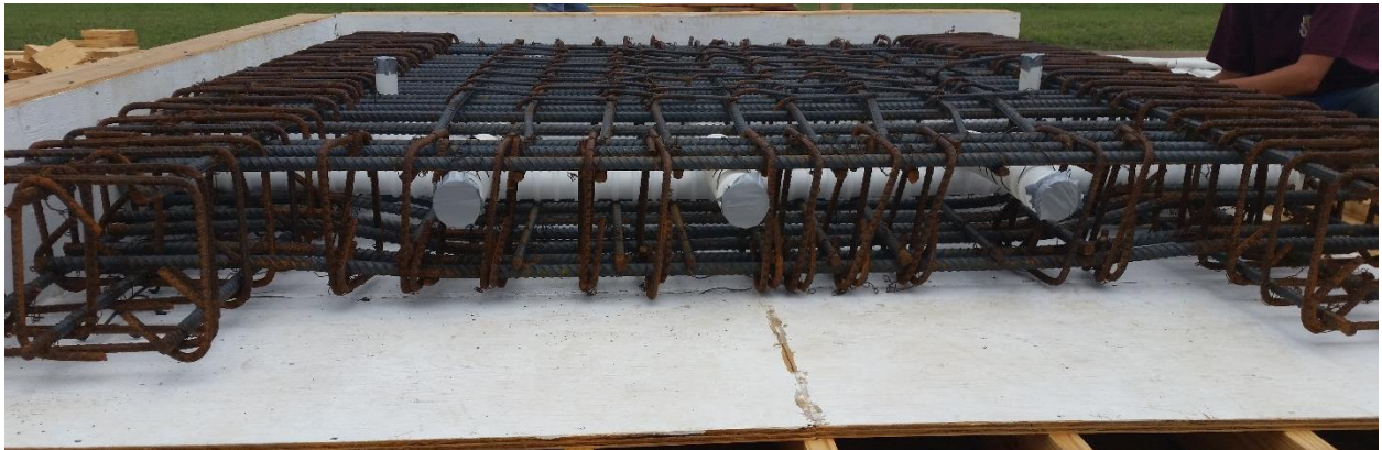
Figure 37 Specimen 1- Post-Tensioning Bar Ducts, Reinforcing Steel Cage, and Formwork View from Between Specimen 1 Feet
