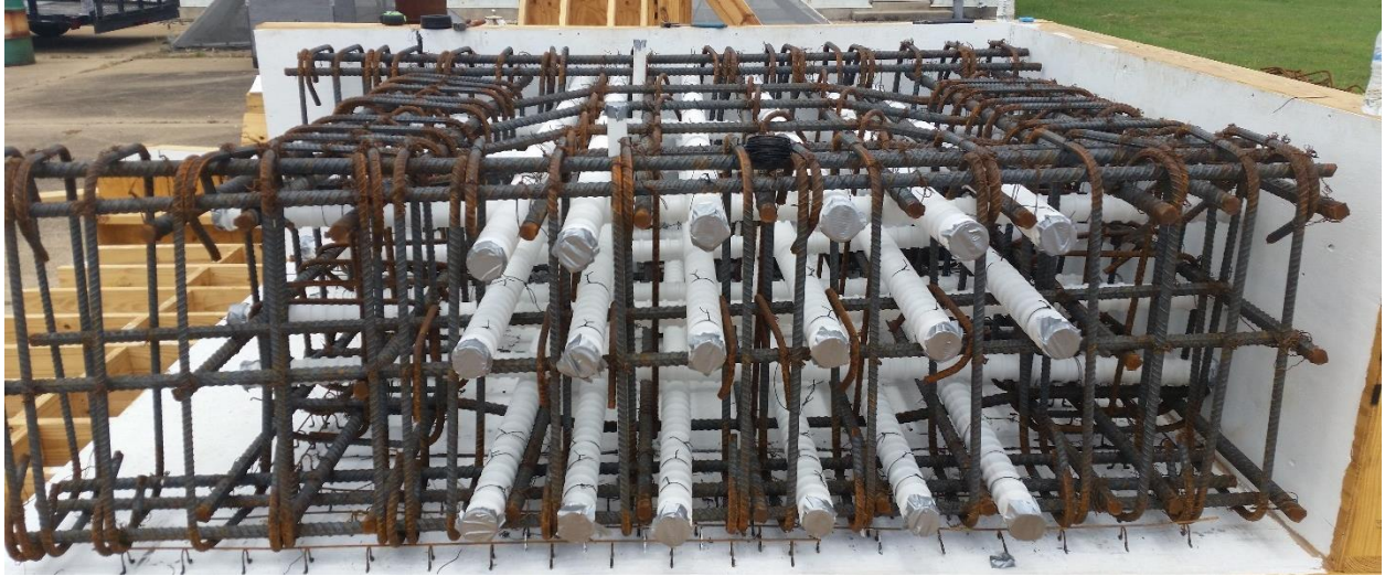
Figure 38 Specimen 2- Post-Tensioning Bar Ducts, Reinforcing Steel Cage, and Formwork View from Side
