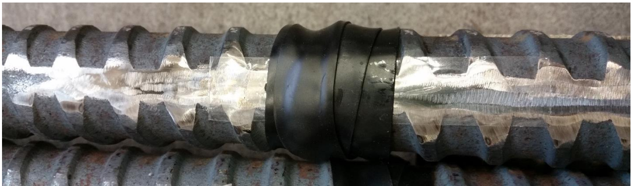
Figure 55 Post-Tensioning Bar with Tape Wrapped Around to Apply Uniform Pressure to Strain Gage for Strong Bond with Adhesive
