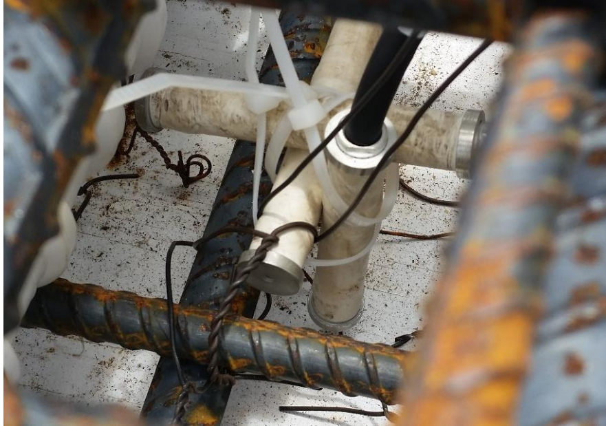
Figure 42 Typical Concrete Gage Installation
