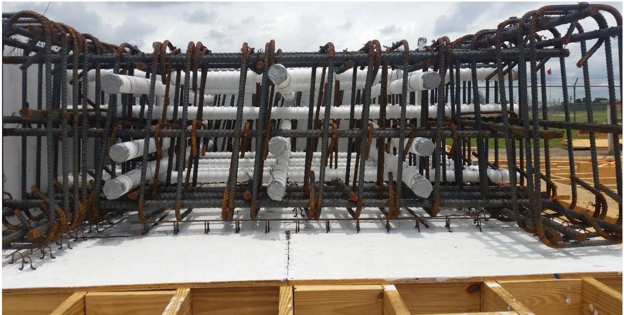
Figure 39 Specimen 2- Post-Tensioning Bar Ducts, Reinforcing Steel Cage, and Formwork View from Between Specimen 2 Feet
