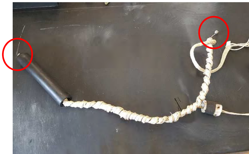
Figure 21. Heating Tape on Fluid Piping
