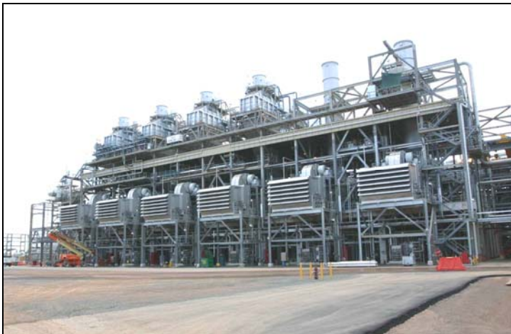
Figure 5. Gas Turbine Compressor Trains with Four Heat Recovery Units (OTSGs) on the left.
