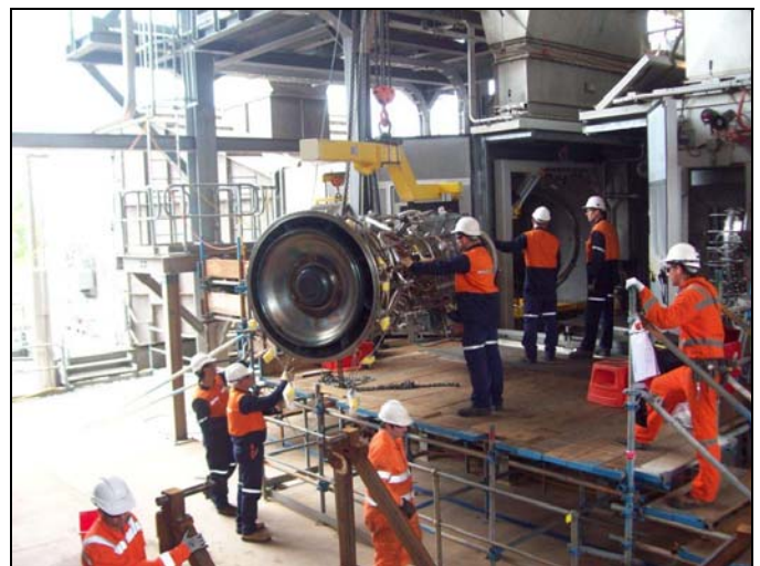
Figure 41. Gas Generator Being Moved into Place for Installation into Enclosure.
