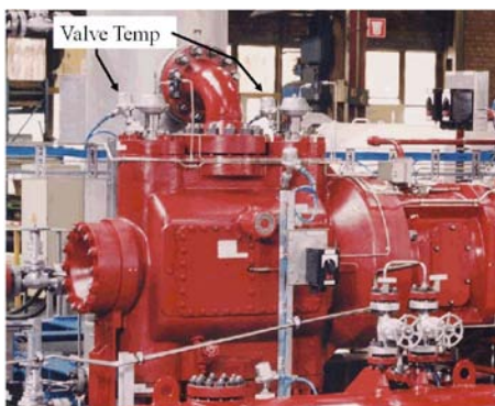
Figure 4: Valve temperature measurement, thermo wells in the valve covers.
