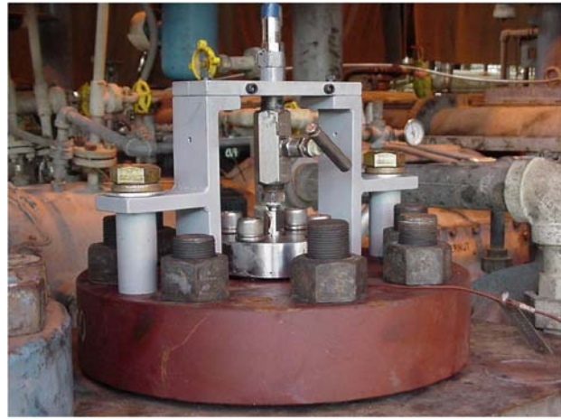
Figure 8: Permanent pressure transducer installation through a valve cover. Courtesy of Bently Nevada.
