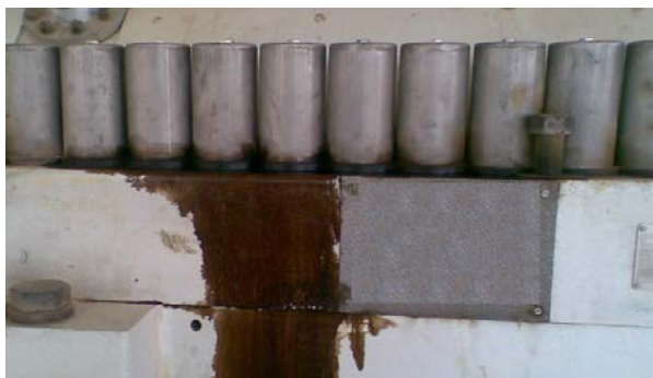
Figure 11. Observed Leakage during operation on site.
