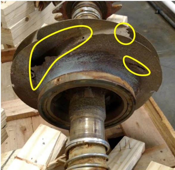
Figure 19. Pump B impeller exhibits cavitation damage from discharge recirculation (yellow).
