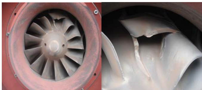
Figure 2: Photographs of failed impeller
