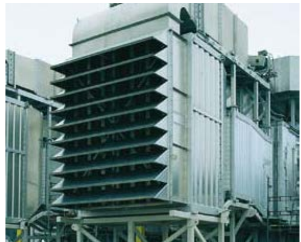
Figure 11. Weather Hood on inlet Filtration System
