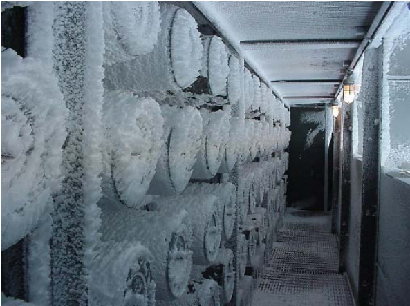
Figure 12. Cartridge Filters with Frost Buildup Due to Cooling Tower Drift
