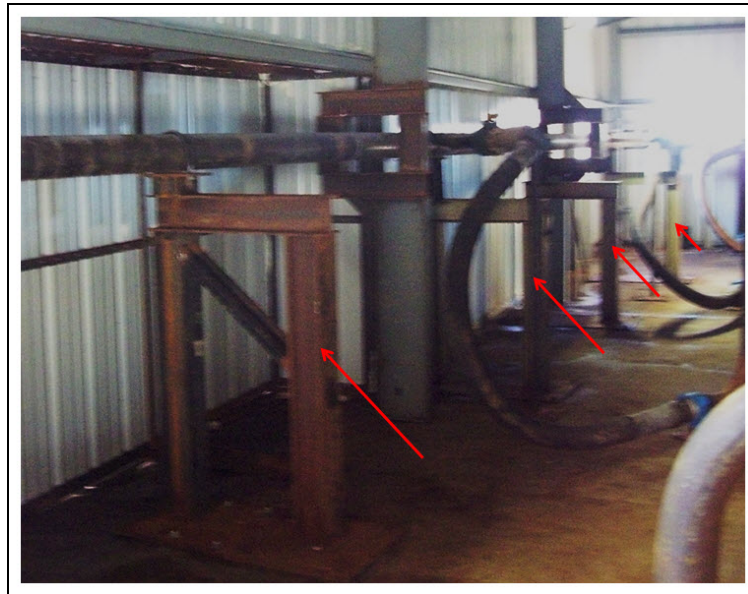
Figure 17: Supports on Header
