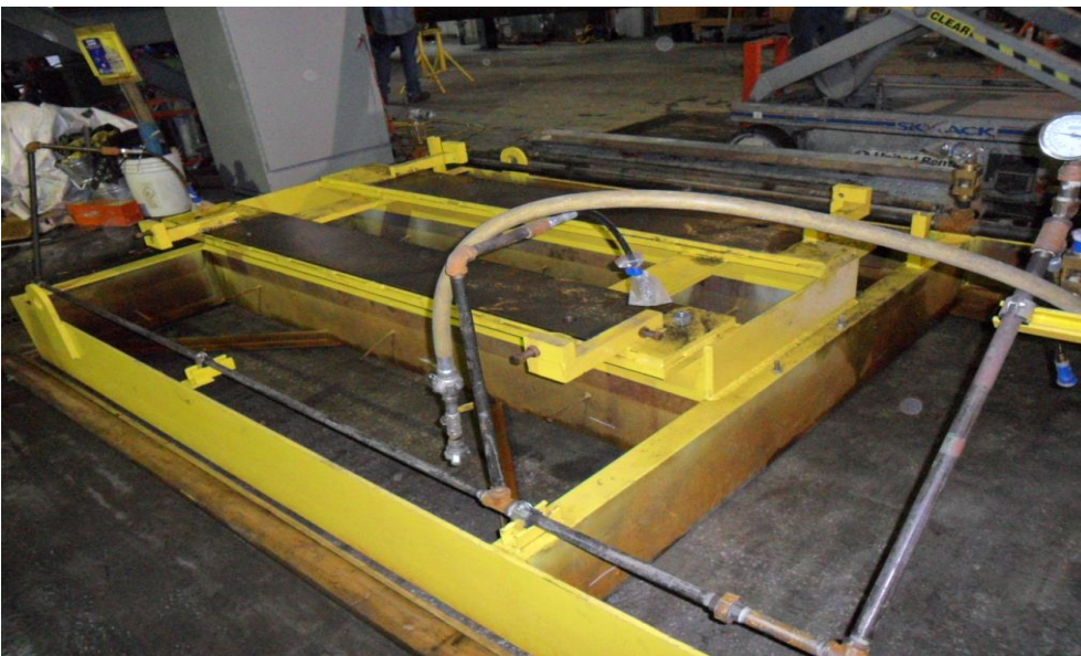
Figure 18: Example of Skid Mounted Equipment
