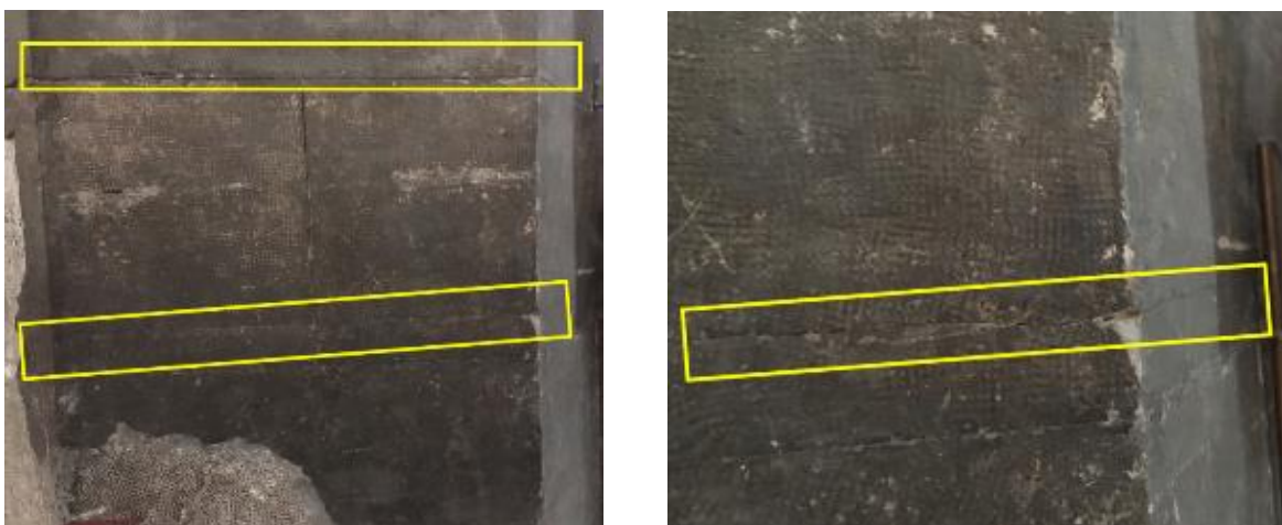
Figure 20: Horizontal cracks in Portland cement repair Pier 2
