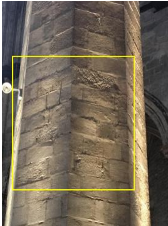
Figure 14: Pitted texture on choir pier
