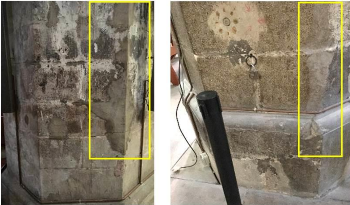
Figure 11: Spalling (left) patched, (right) unpatched
