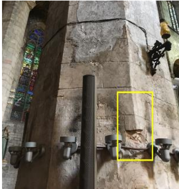
Figure 19: Cracks and spalls in Portland cement repair
