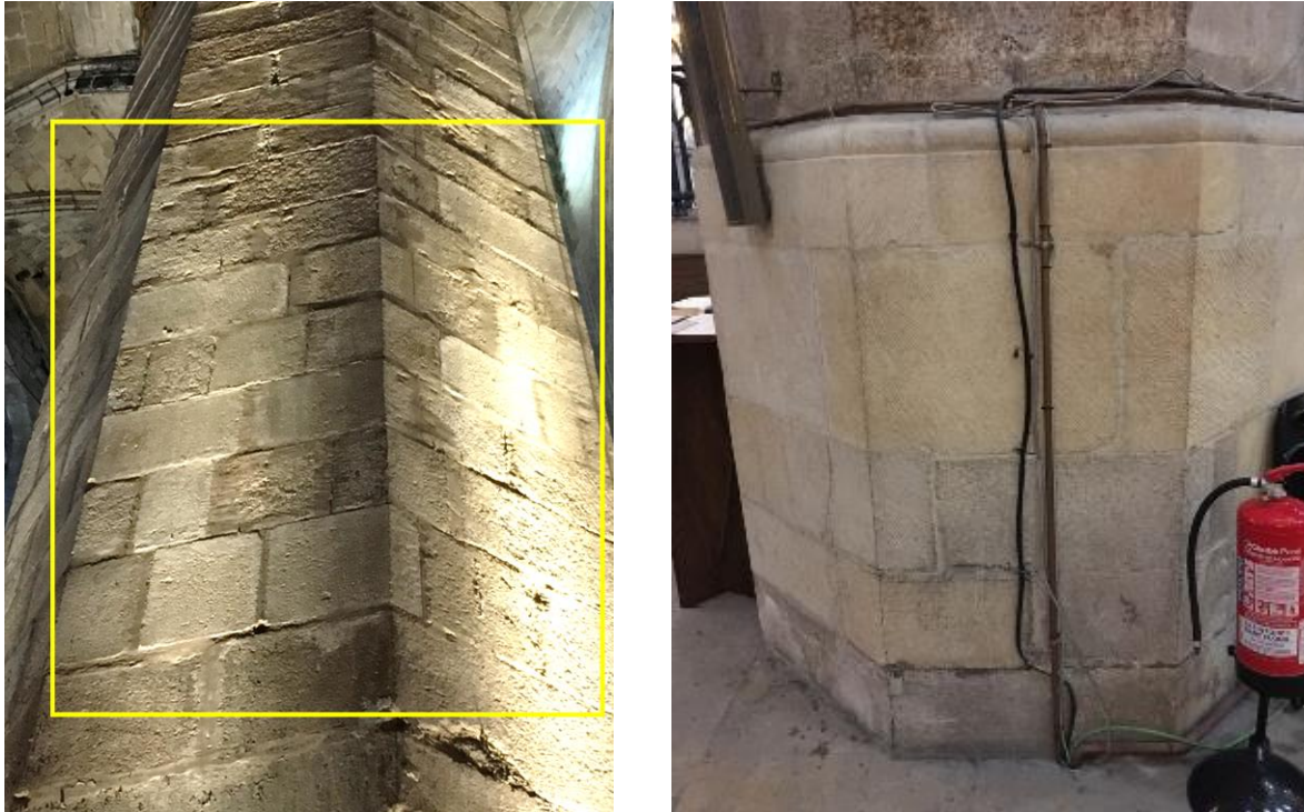
Figure 18: Stone replacements in choir (left) mid-height, (right) base
