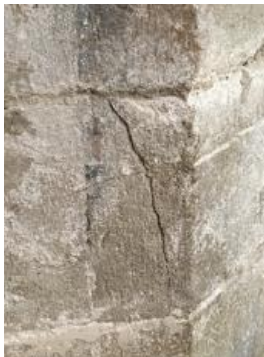
Figure 8: Single block crack
