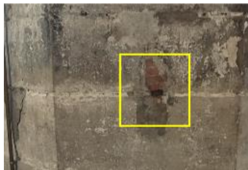
Figure 23: Brick mount with corroded iron
