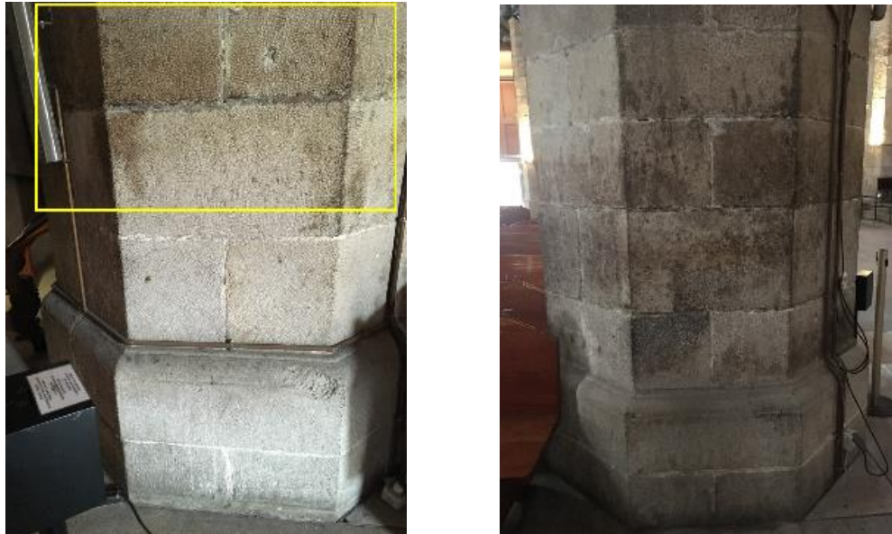
Figure 15: Speckled staining (left) Pier 1, (right) Pier 8
