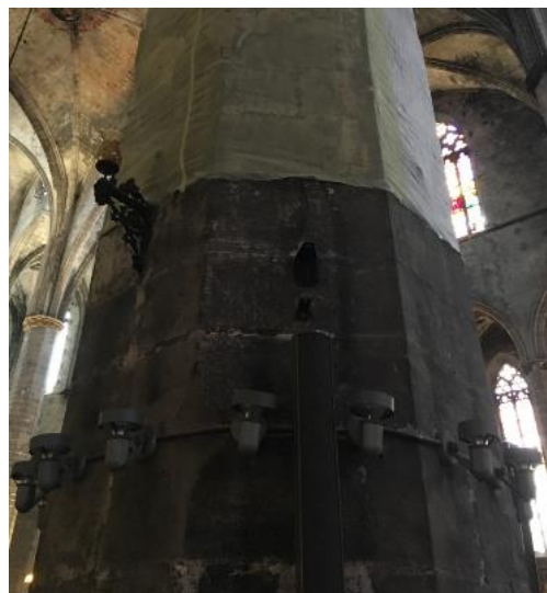
Figure 16: Soot accumulation on Pier 7
