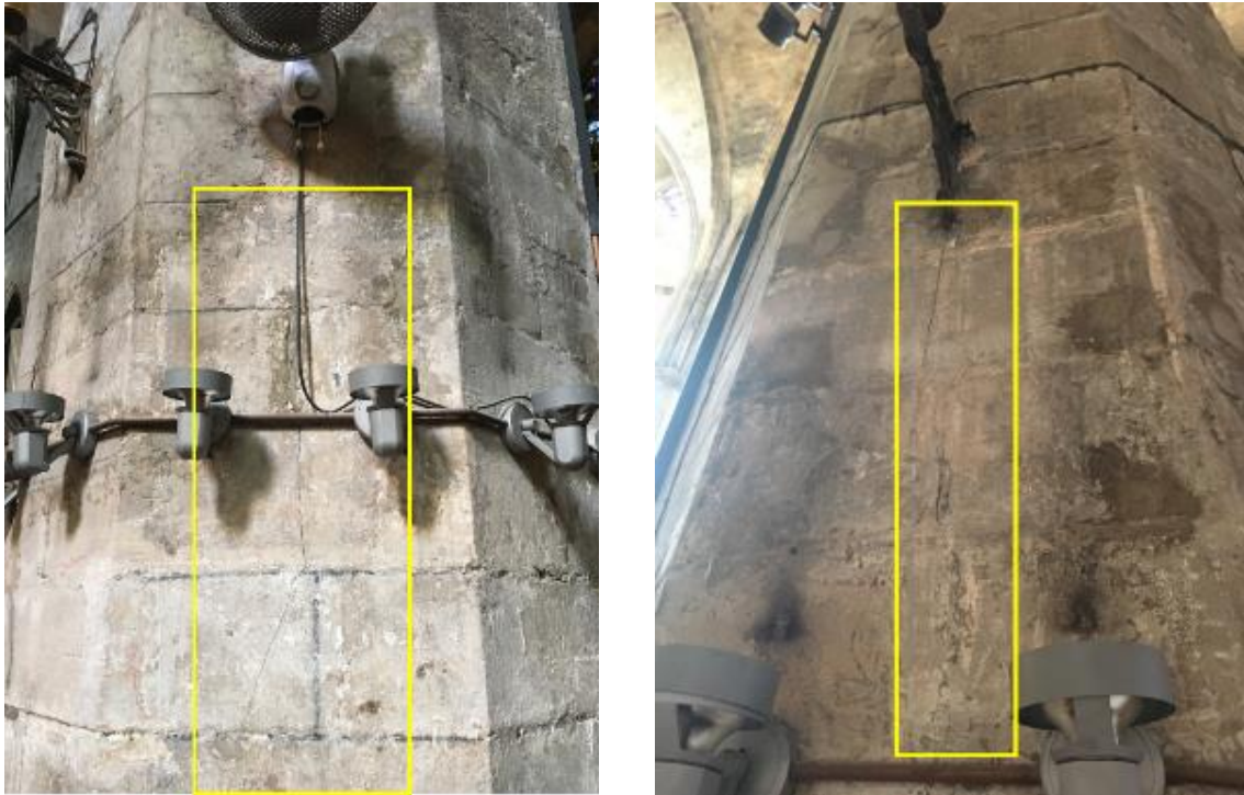
Figure 22: Cracks below fixtures
