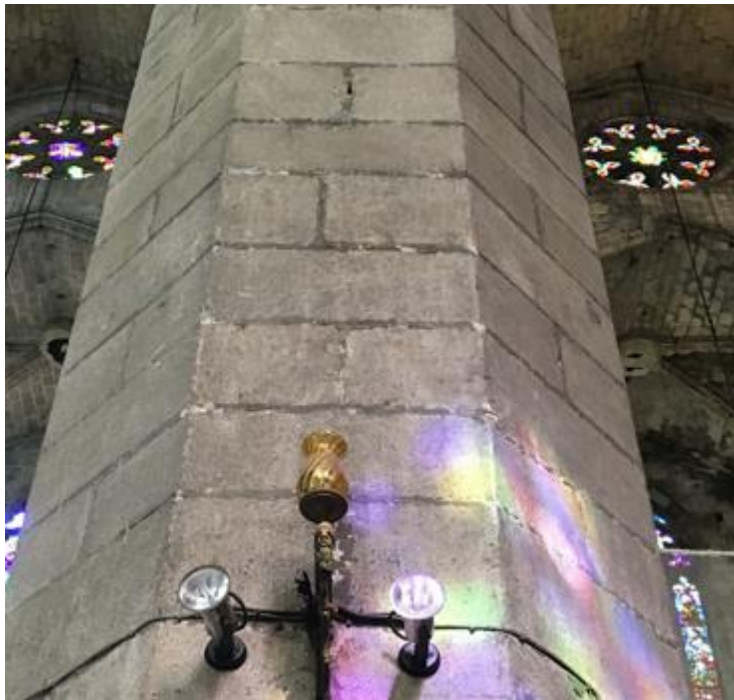
Figure 17: Joints repointed with Portland cement mortar (note darker color)
