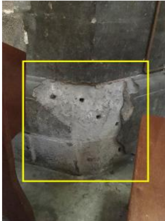
Figure 21: Crusting of repair at base
