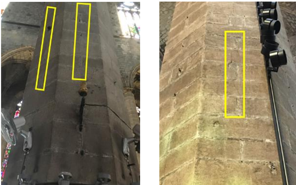
Figure 9: Multi-block vertical cracks (left) shows successive faces
