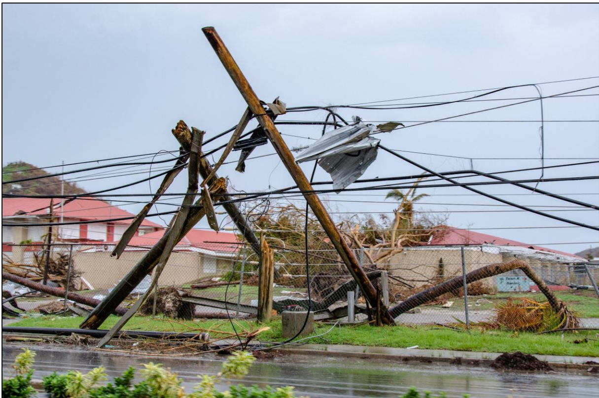
Figure 5. Snapped utility poles in St. Thomas, U.S. Virgin Islands, after Hurricane Irma
