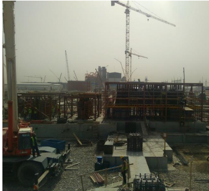
Figure 8.9 Electrical power station – Besmaya – Phase 2, Baghdad, Iraq [© Denco Structural Engineering P.C.]
