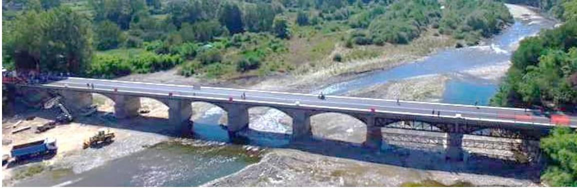
Figure 10.33 Repair, rehabilitation and seismic upgrading of an existing historical masonry bridge damaged by flooding [© reprinted with author's permission]
