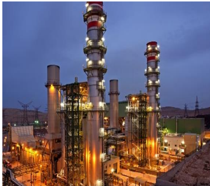
Figure 8.12 ZARQA PHASE III ADD-ON CCPP, Zarqa, Jordan [© DENCO Structural Engineering P.C.]
