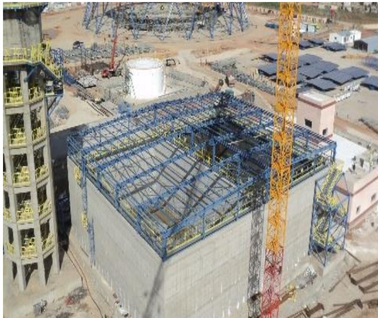
Figure 8.13 DEIR ALI II CCPP, Deir Ali, Syria [© Denco Structural Engineering P.C.]
