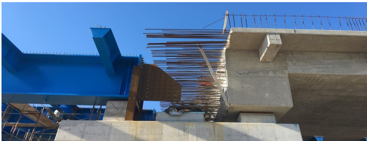
Figure 8.18 Joint between central and lateral spans of the new Kamares Bridge (south branch), before continuity is achieved [© DENCO Structural Engineering P.C.]
