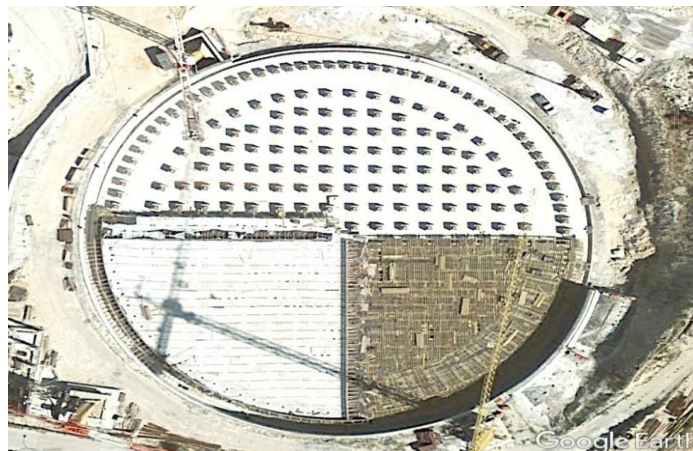
Figure 8.23 View of the triple FPS base isolators of the 3 rd LNG Reservoir in Revythousa island, Greece, during construction [© DENCO Structural Engineering P.C.]
