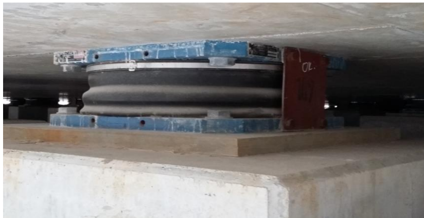
Figure 8.22 Triple FPS used for the seismic isolation of the 3 rd LNG Reservoir in Revythousa island, Greece [© DENCO Structural Engineering P.C.]
