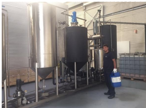
FIGURE 14 - PILOT PLANT AT GRUPO SOUSA / METAL LOBOS LDA.
