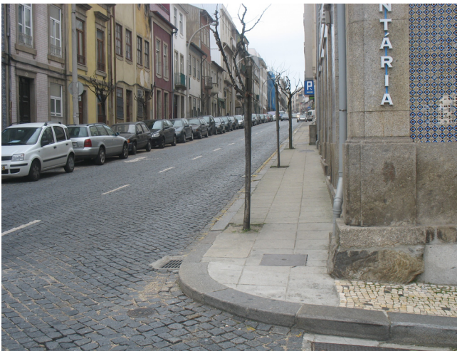
Figure 4: Poorly maintained width of sidewalks in Braga.
