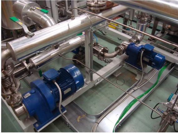
Figure 4.4 -P8 (left) and P2 (right) circulating pumps.
