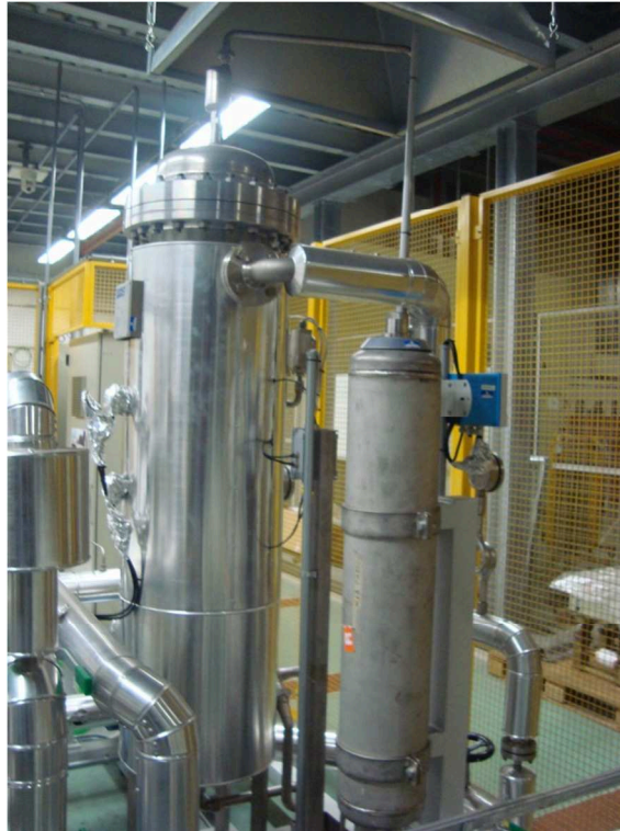
Figure 4.8 - Boiler (left), pressurizer (right) and safety aspiration gate (above).
