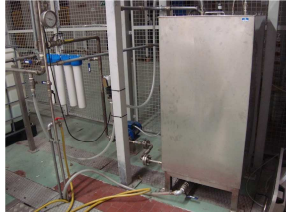
Figure 4.5 - Electro polished stainless steel reservoir and four purification modules for water deionization process.
