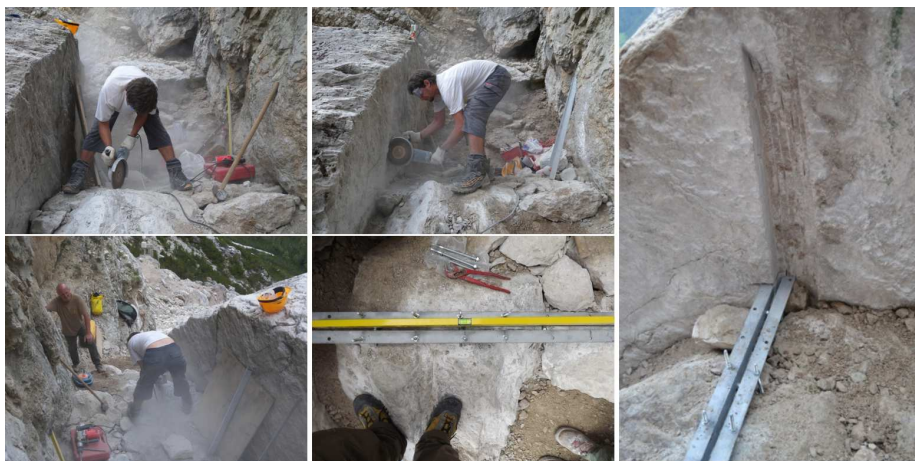
Figure A.4: Building of the facility (August 2011): rock cutting for positioning the steel plate.
