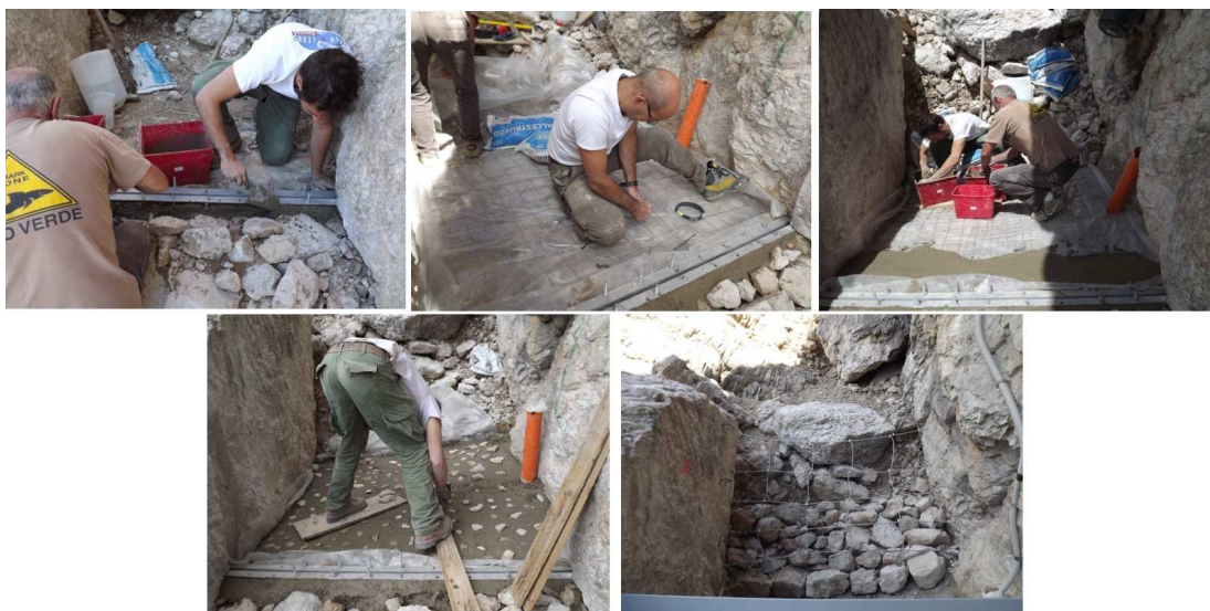
Figure A.5: Building of the facility (August 2011): preparation of the upstream basin.
