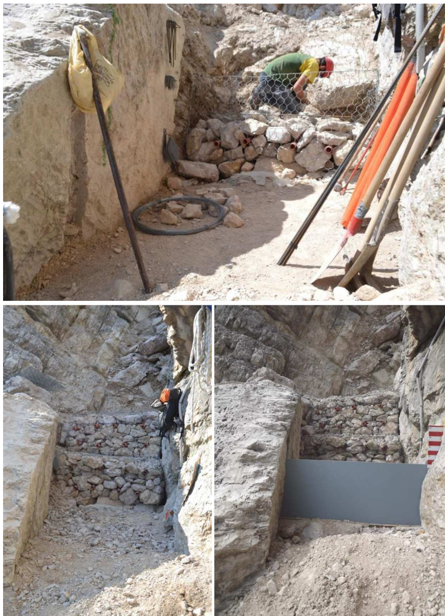
Figure A.8: Re-positioning of the sharp crested weir. The upper panel exhibits the building-up of the gabions upstream the stilling basin. The lower panels show the finished stilling basin, without/with the sharp-crested weir (respectively on the left and the right).
