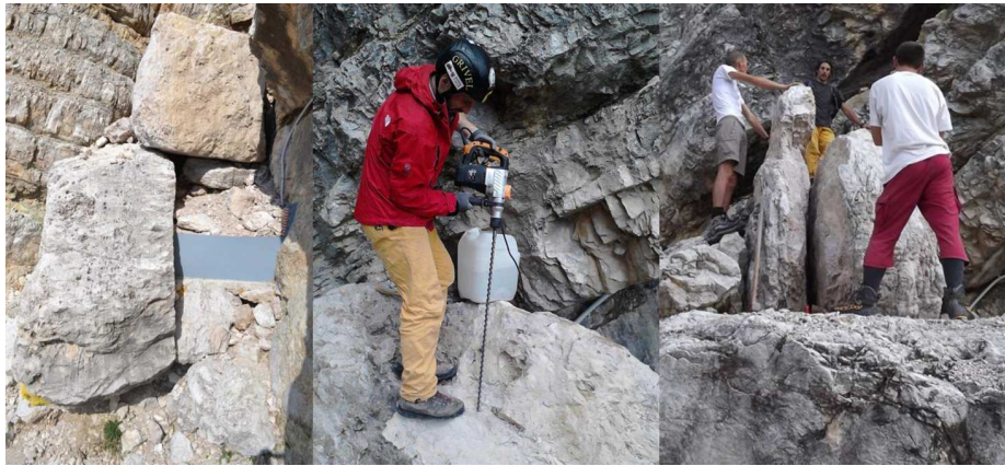
Figure A.6: Removal of the huge boulder obstructing the facility. On the left, the situation found after the rockfall occurred on August 2011; the central panel shows the drilling of the huge boulder above the stilling basin for using the expansive mortar; on the right, the cracked boulder, before removal.
