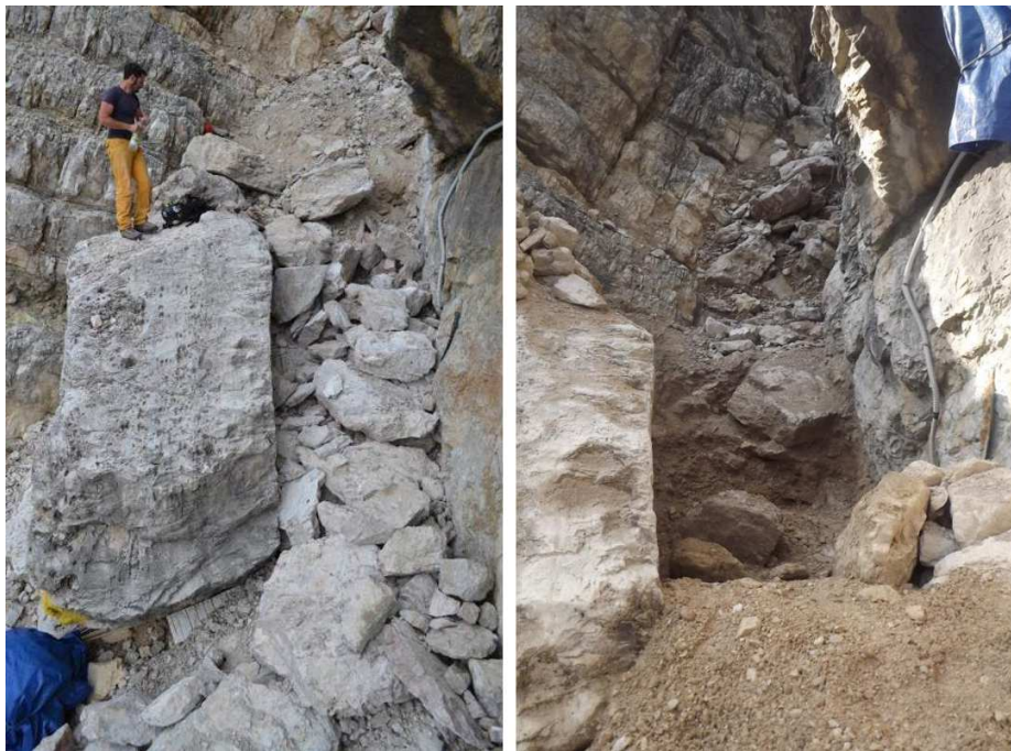
Figure A.7: Consolidation of the torrent bed. On the left, the channel after the removal of the huge boulder; on the right, the dug channel before building the gabions upstream the stilling basin.
