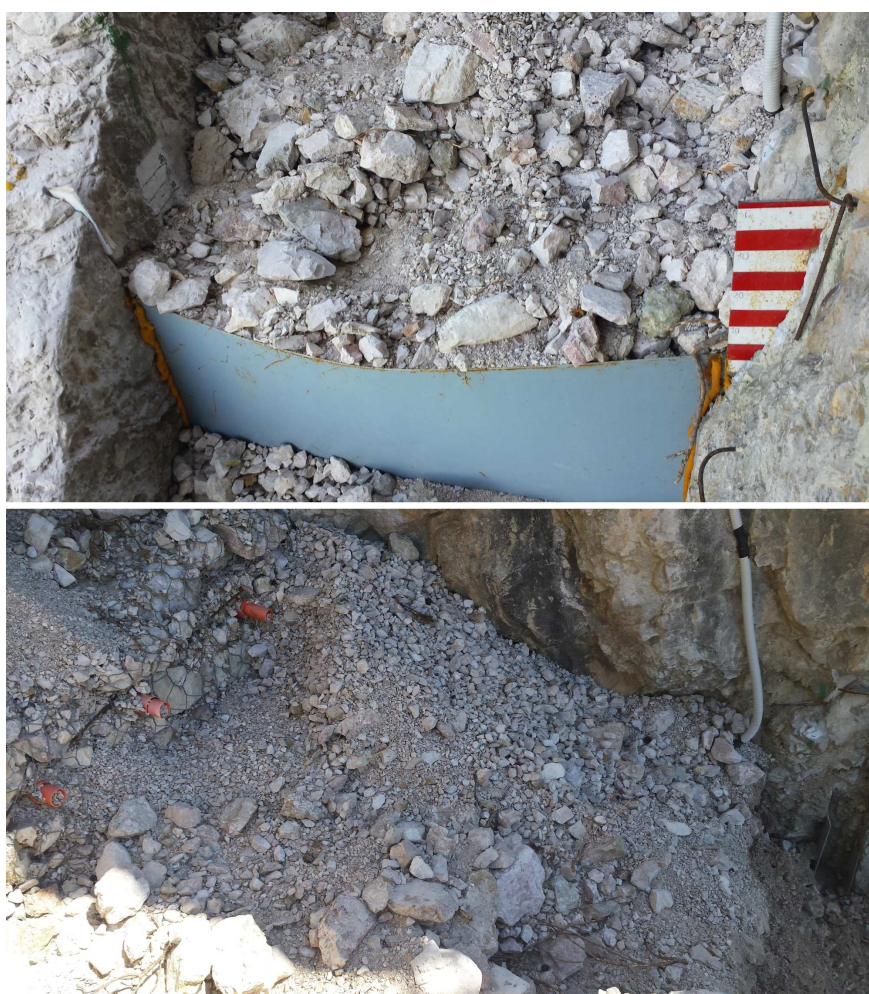
Figure A.10: Stilling basin after the sediment transport events occurred on June 7 th (upper panel), and on July 29 th , 2015 (lower panel).
