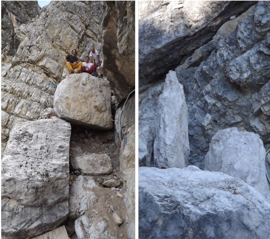
Figure 2.5: On the left, the situation found after the rockfall occurred on August 2011; on the right, the cracked boulder, before removal.
