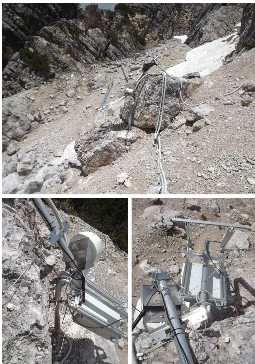
Figure A.9: Monitoring station after the repeated snow avalanches occurred during Winter 2014.
