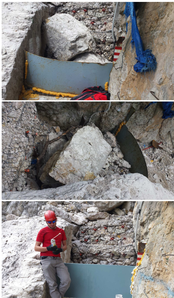
Figure A.11: Stilling basin before starting the monitoring season on 2016 (upper and central panel). In the lower panel, the restoration of the facility, with the replacement of the damaged sharp-crested weir.
