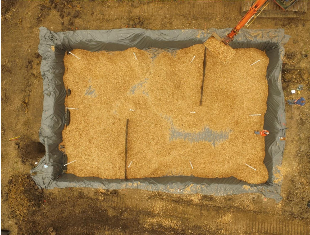
Figure 7. Aerial image of the Advanced Bioreactor detailing the well and baffle placement before the geofabric and soil cap was placed during construction.
