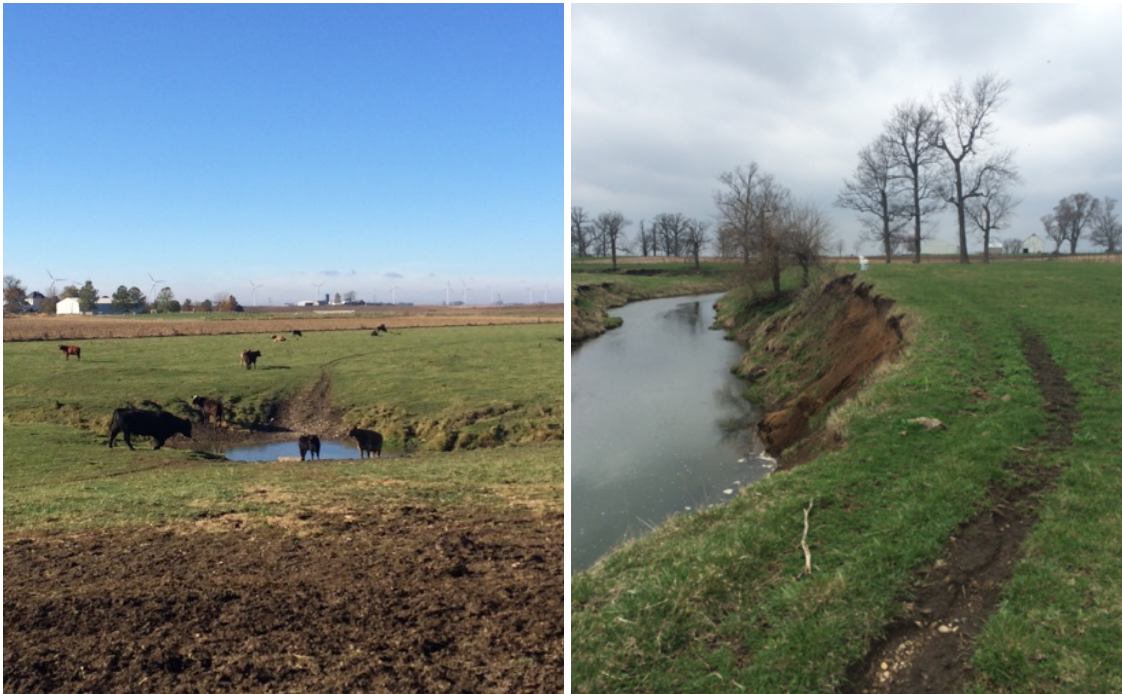
Figure 2.10: (Left) Bare soil (foreground) from cattle trampling on a floodplain surface with unvegetated cattle ramp in background. (Right) Eroded streambank and unvegetated cattle pathway.
