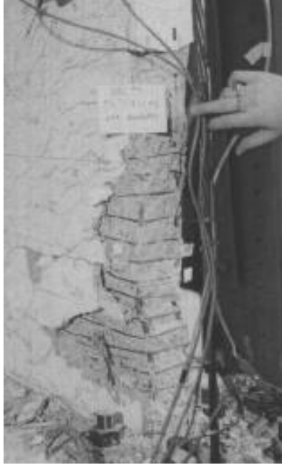
Figure 2.17: Specimen TW2 web failure (Thomsen IV and Wallace 2004)
