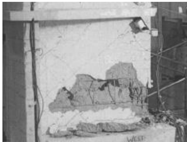
Figure 2.16: Specimen TW1 web failure (Thomsen IV and Wallace 2004)
