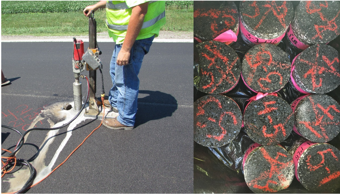
Figure 7-6 Core extraction at the location of GPR measurement (left), and cores taken (right)
