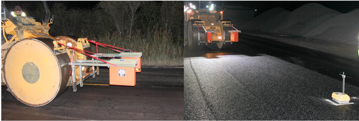
Figure 8-9 AC pavement compaction monitoring using GPR on the leveling binder (left) and the SMA surface (right)
