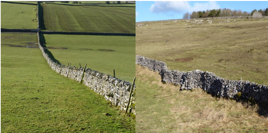
Well-maintained stock-proof wall (left). Bellying walls close to Roystone Grange (right).
