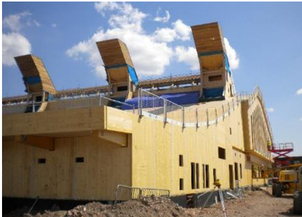
Figure 6: The 'carbon neutral' GlaxoSmithKline (GSK) Sustainable Chemistry Building, University of Nottingham, UK, under construction, 24th July 2014, which has predominantly timber structure and cladding above ground [Photograph ©John Chilton]
