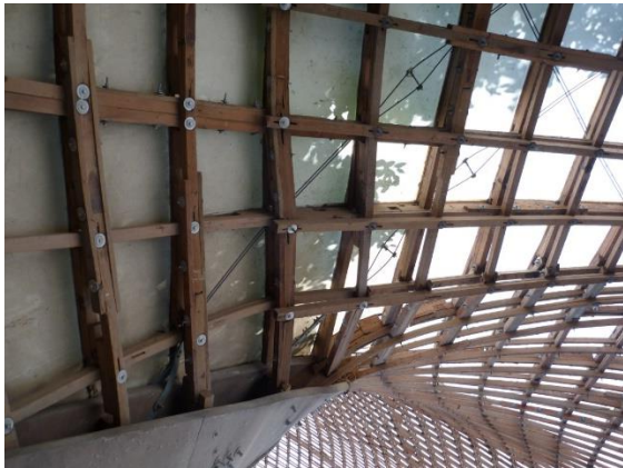
Figure 12: Mannheim Multihalle was restrained by a diagonal network of twin 6mm diameter stainless steel wire ties installed at 4.5m centres. (Happold and Liddell, 1975) after the gridmats were pushed up from the ground. [Photograph © Gabriel Tang]
