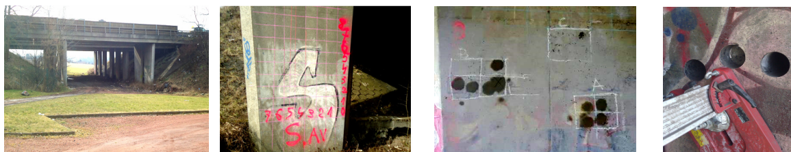
Figure 4: Tests on a highway bridge in Marly A: Structure B: Pre-auscultation grid C : Auscultation zones D :Coring
