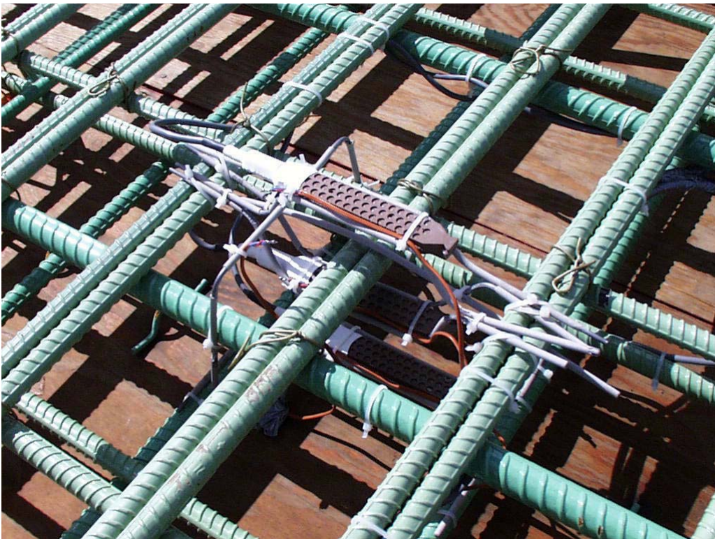
Figure 222. Sensor location A, over pier No. 4, center of deck, L. Springfield
