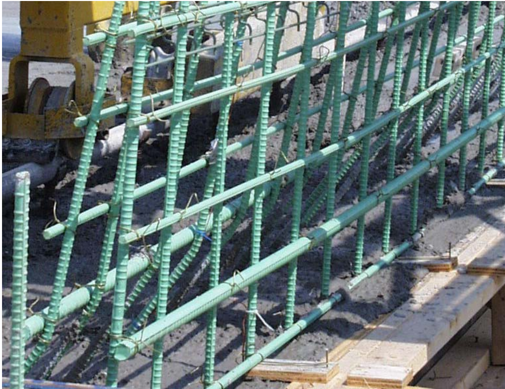
Figure 135. Sensors installed in parapet wall
