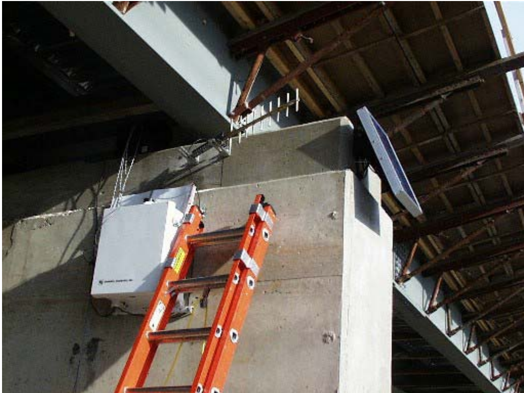
Figure 127. Complete installation with solar panel and cellular antenna
