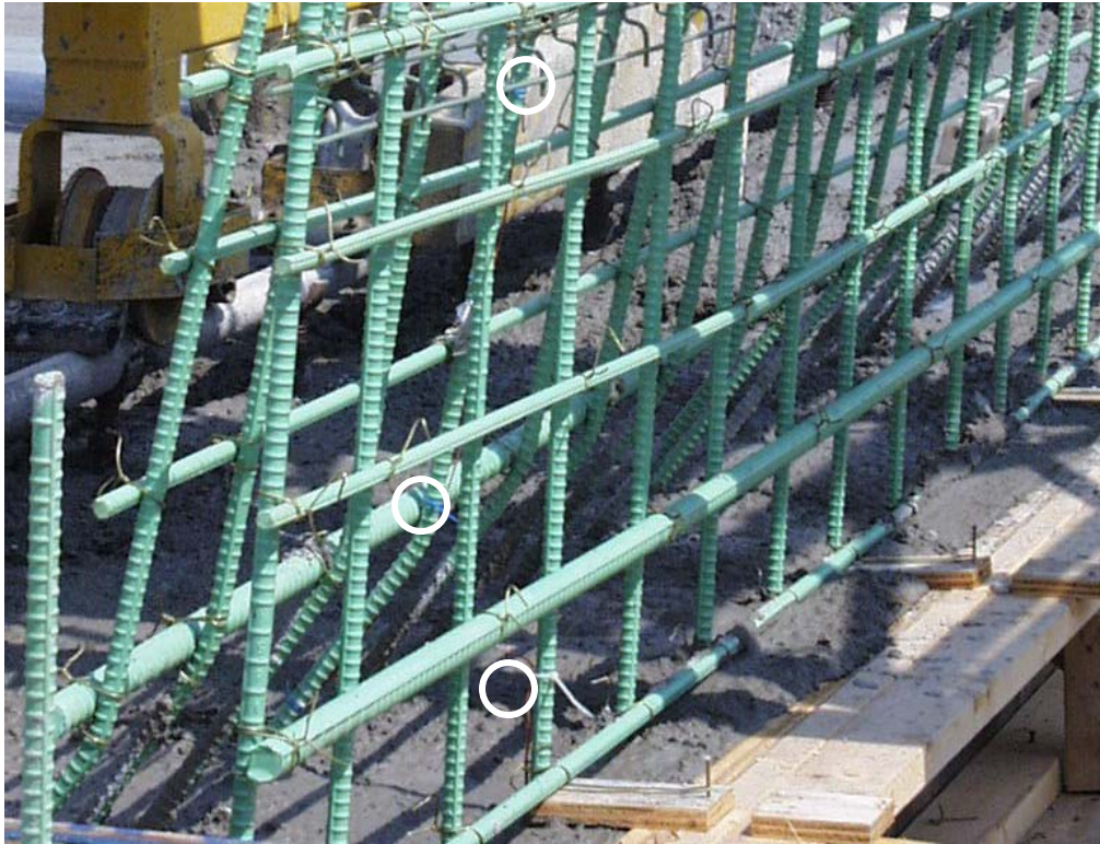
Figure 237. Sensors installed in parapet wall, Big Creek
