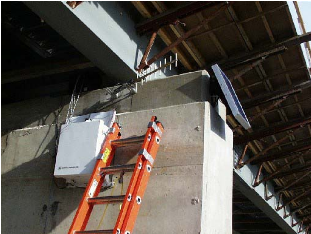
Figure 211. Complete installation with solar panel and cellular antenna, Duncan Rd.
