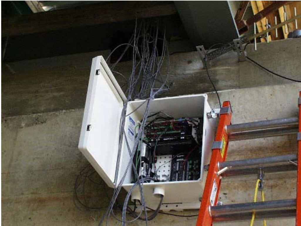
Figure 210. Data collection equipment during installation on pier at Duncan Rd
