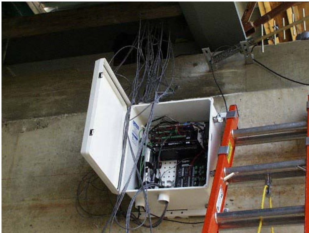
Figure 126. Data collection equipment during installation on pier at Duncan Rd
