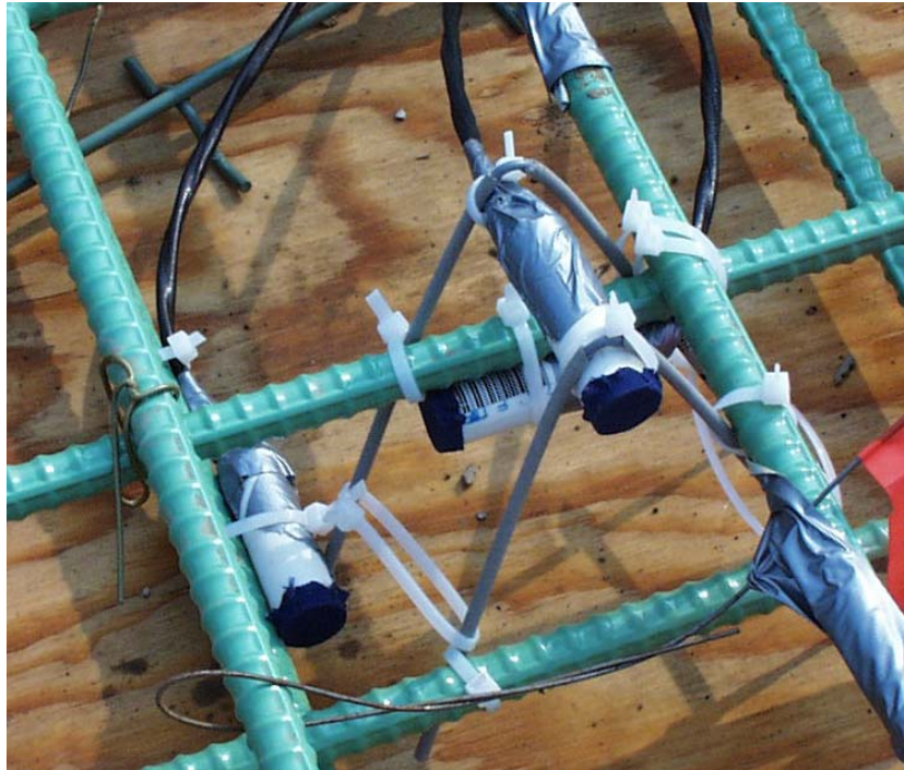
Figure 260. Internal RH sensors mounted for casting in concrete bridge deck, Big Creek
