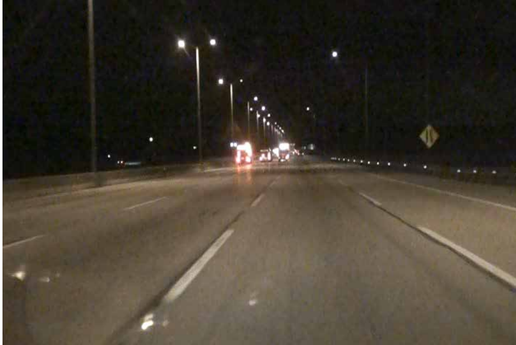
Figure 6.9 A nighttime maintenance operation on an urban expressway. The left shoulder and two left lanes (of four traffic lanes) are temporarily closed for maintenance.
