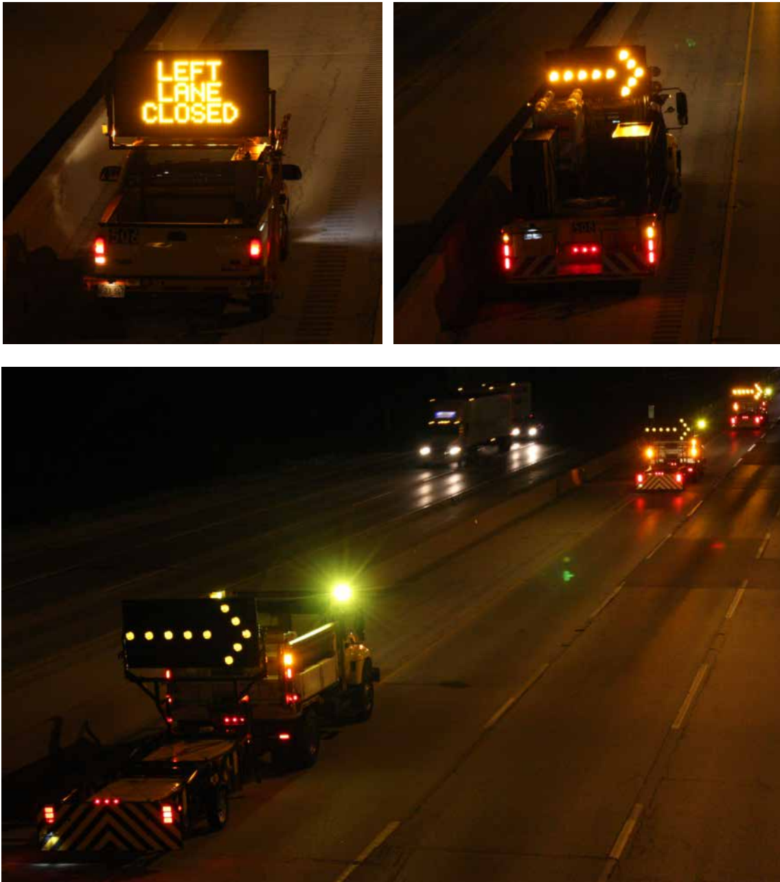
Figure 4.3 Vehicles and equipment used for the mobile lane closure on I-90 near the Des Plaines Oasis.
