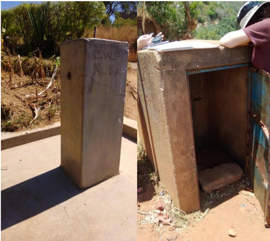
Figure 26 Abandoned tap in Ronge on the way down to Mwatate from Chawia. In the neighbourhood there is also a water tank, funded by Danida that has never contained water. (Kivivuori 2013)
