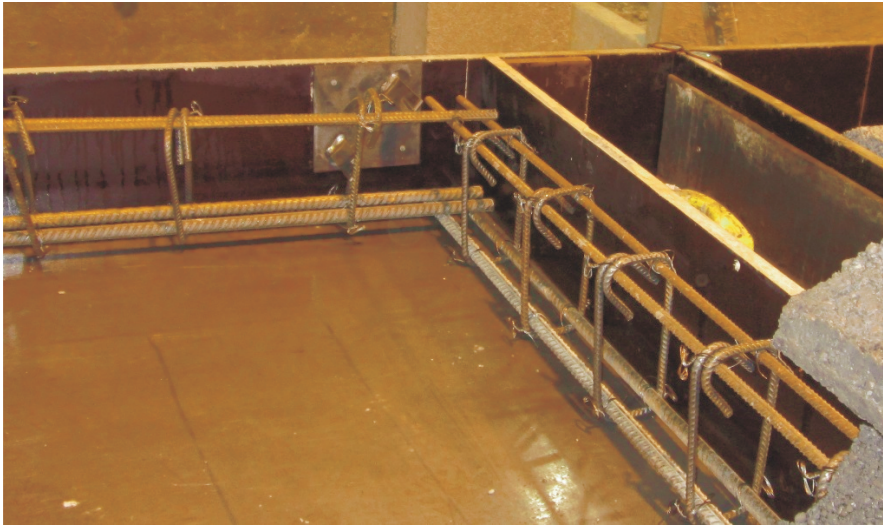
Figure 4: Beam reinforcement placed in order to create edge and end beams in a super-light element
