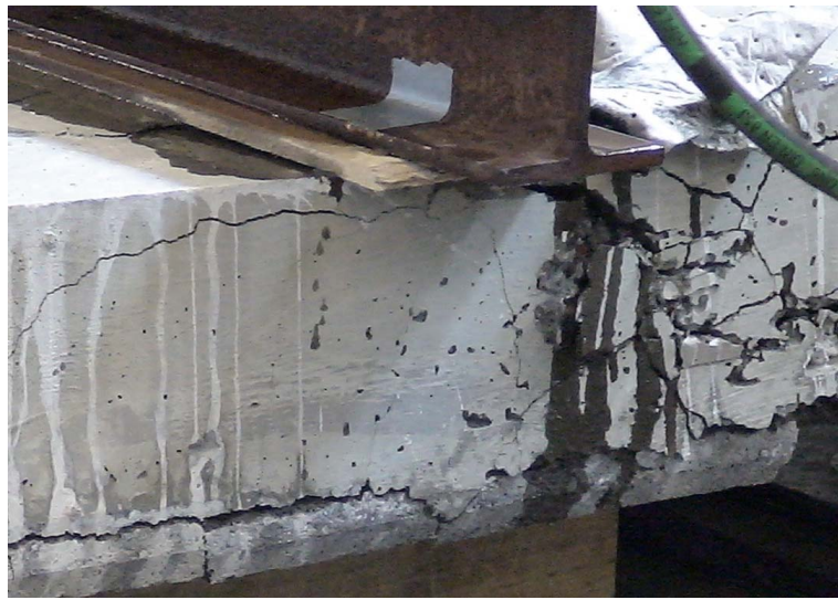
Figure 4.5: Cracking development in the super-light slab element tested in bending, the wet area is leaked oil from the oil press.
