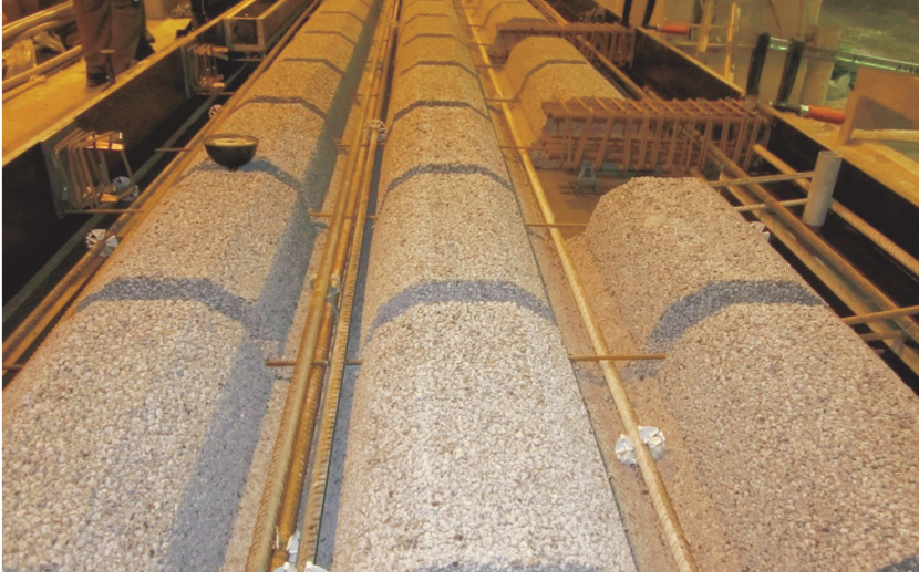
Figure 5: Super-light element with LWAC blocks and reinforcement prior to normal concrete being cast
