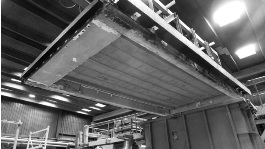
Fig. 14- Unharmed SL-Deck after 135 min standard fire exposure with 17.6 kN/m 2 (367 lbf/ft 2 ) load.
