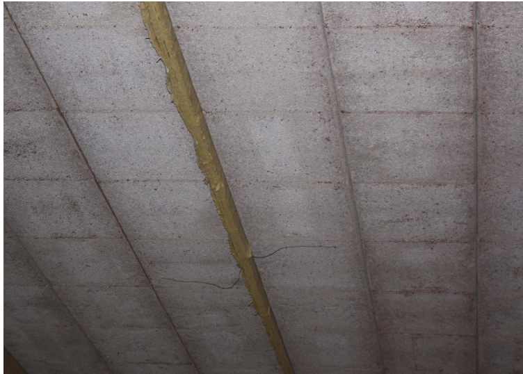
Figure 4.9: View of the element used for the fire test from below after the test.
