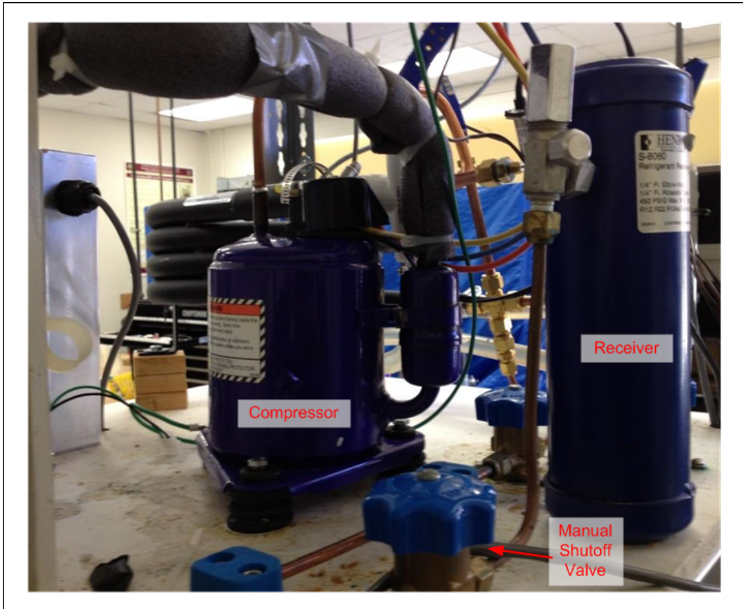
Figure 2.9: Photo of compressor, liquid receiver, and manual shutoff valve
