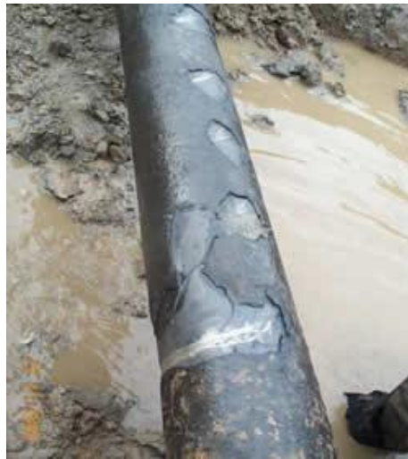
Figure 1: Pipeline Damaged by an Excavator [3]
