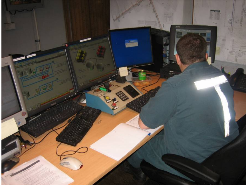
Figure 2 A typical mining control room (see online version for colours)
