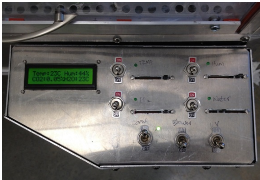
Figure 28: Assembled Control Panel
