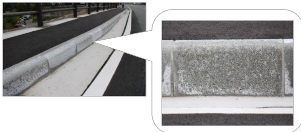
Figure 1 – Degraded GP walkway boundary block placed on strongly acidic soil (Beppu Myoban Spa, Oita, Japan)
