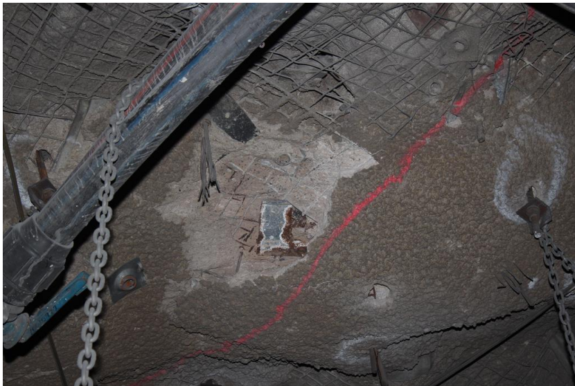
Figure 18 - Loss of adhesion leading to ejection of small blocks of shotcrete from the excavation roof, influenced by reinforcement surface fixtures.
