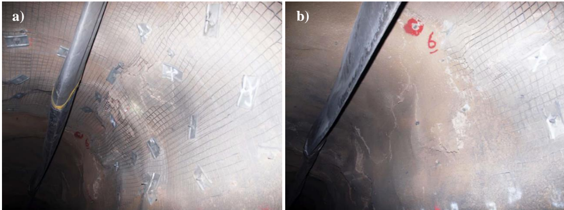
Figure 12 – a) Fibre reinforced versus b) mesh reinforced shotcrete displacement observations indicate superior surface support performance when mesh is embedded in shotcrete, rather than being installed externally.
