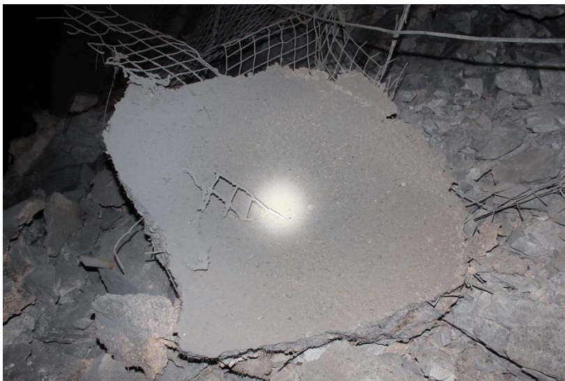
Figure 16 – Mesh reinforced shotcrete failure in a rectangular block of a size defined by the reinforcement pattern following extreme energy demand ( >50\text{kJ/m}^2 ).
