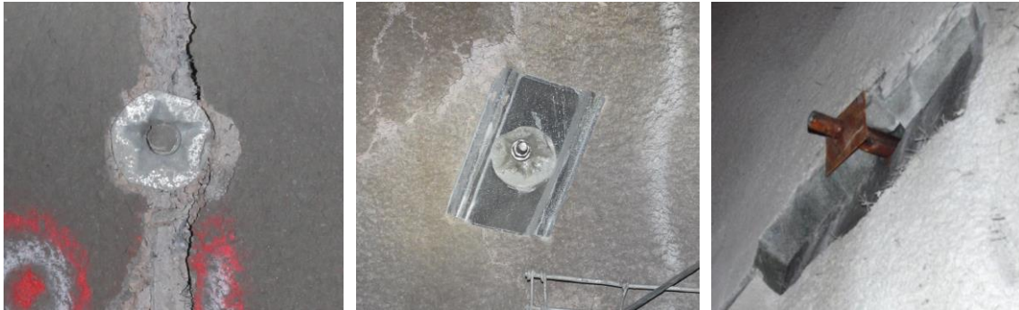
Figure 6 – Plates provide limited load transfer between shotcrete and reinforcement.
