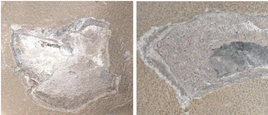
Figure 5 - Compressive failure of shotcrete, also known as shotcrete spalling.
