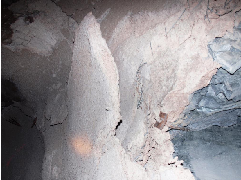
Figure 17 - Loss of adhesion between primary and secondary shotcrete layers leading to formation of unstable blocks in the wall.
