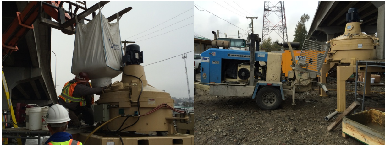
Figure 1: Concrete pan mixer and wet-mix shotcrete pump. After mixing, shotcrete was discharged into the shotcrete pump.
